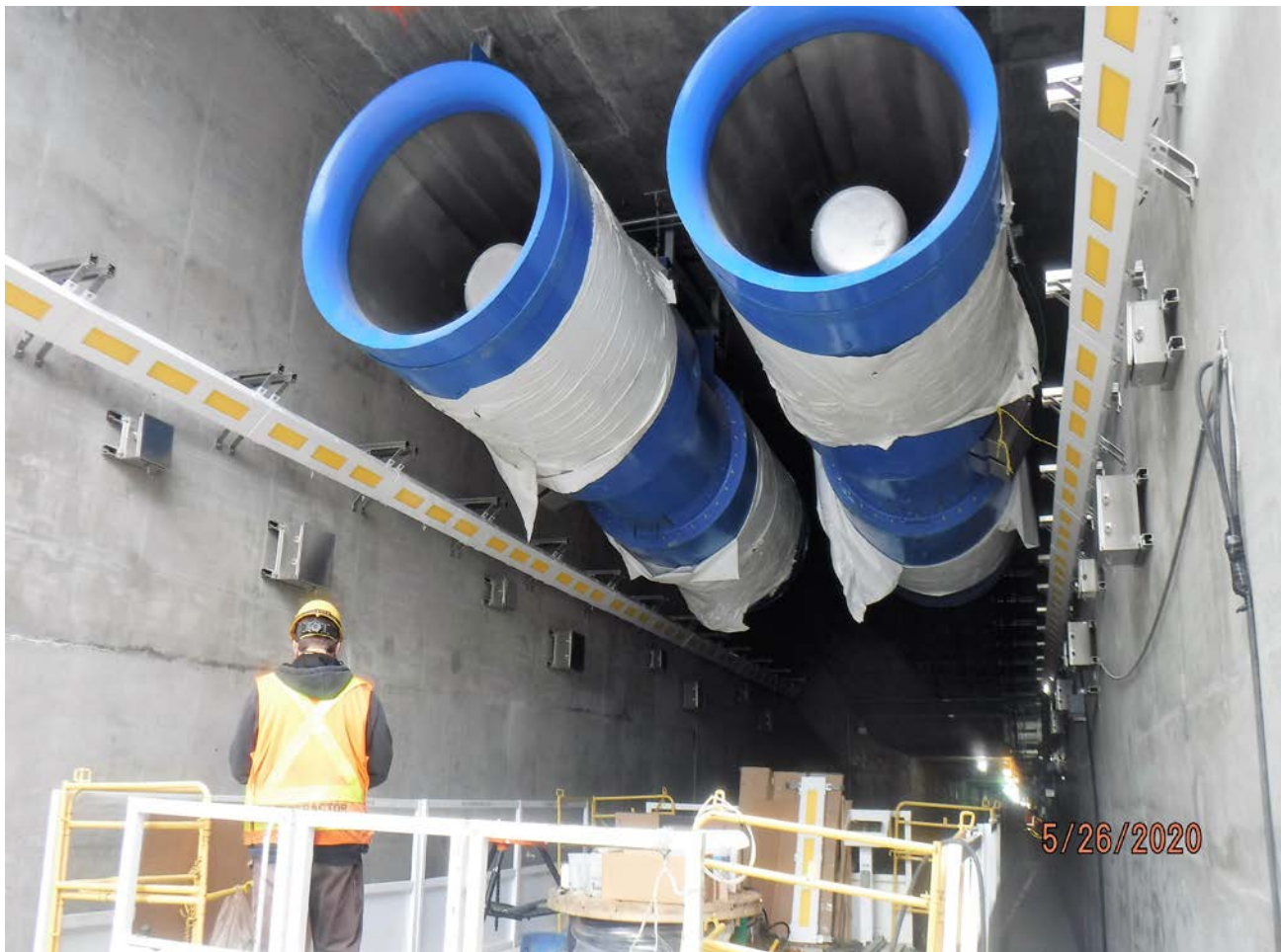
The picture above depicts the layout and installation of tunnel lights in one of the approach structures in Queens. The work is being performed under the CS179 contract.
