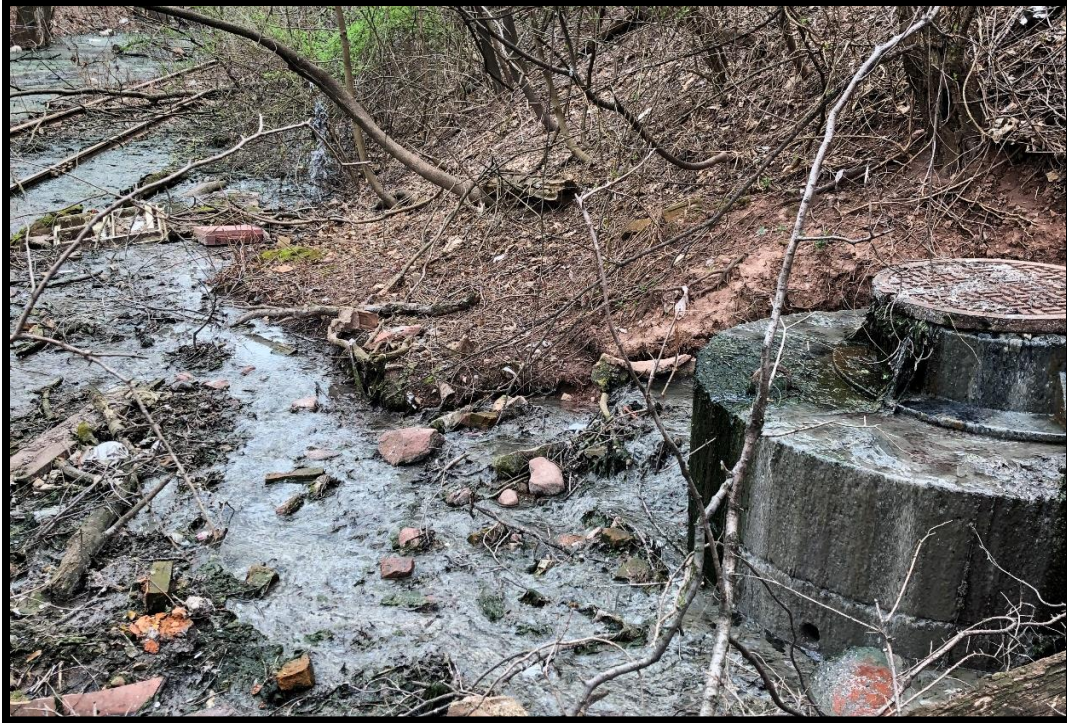
Photo O: View of a leaking sewer depositing water into the recessed portion of the study area near Lake Avenue.
