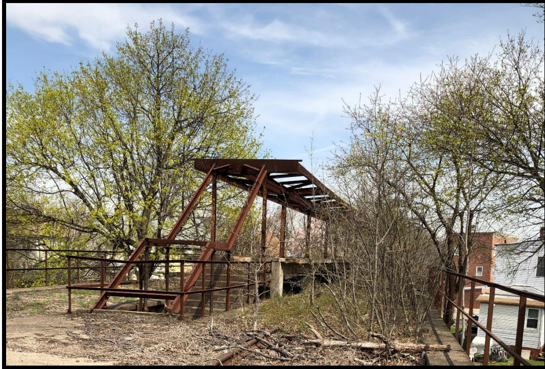
Photo S: View looking at mid successional species colonizing the elevated platform near the Port Richmond station platform.
