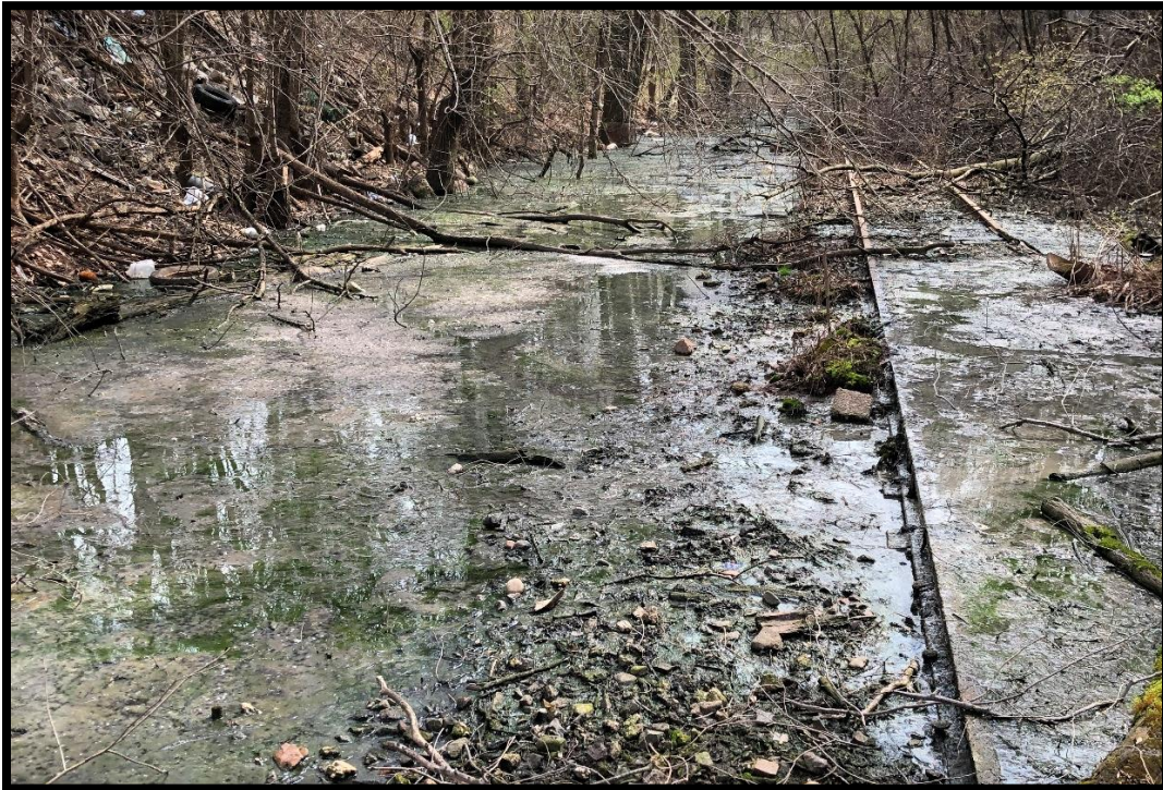
Photo P: View looking east at pooled sewer water resulting from the leaking sewer system this area appears to lack any wetland characteristics and is underlain by ballast and gravel.
